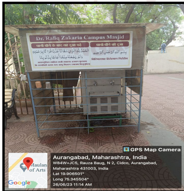
Drinking Water Facility
